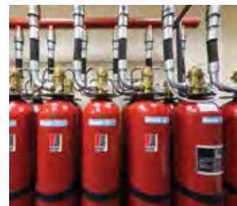
FM-200 GAS EXTINGUISHING SYSTEM
