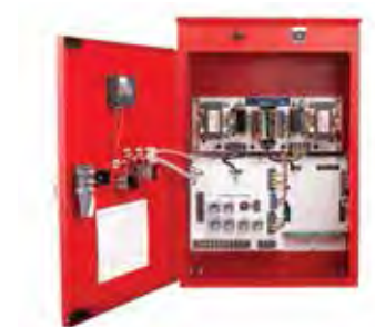
FIRE PUMP CONTROL PANEL
