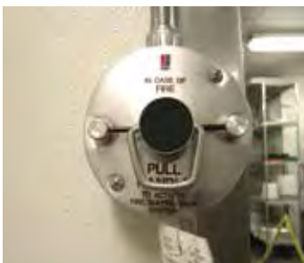
KITCHEN HOOD SYSTEMS
